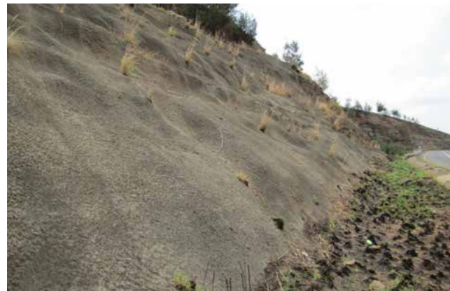
Photo 7a: Steep embankments in weatherable rock like slaking shale can be sealed with shotcrete. (Oliviershoek Pass shotcreted some 40 years ago.)
