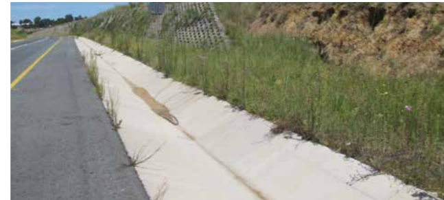
Photo 8: Steep embankments in soft material can be protected with one or other form of retaining wall.
