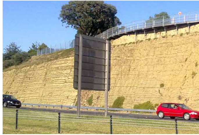
Photo 6: A cut embankment in hard poorly weatherable rock is best cleaned and left bare. Geological strata are an interesting feature of our heritage, and there is no harm in proudly exposing them.
