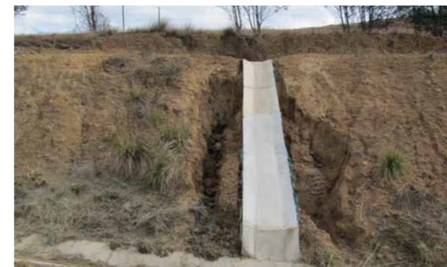
Photo 3: Roads are ‘permanent’ infrastructure. During their long life they will experience extreme events, and should therefore be designed accordingly. This design is a candidate for Justice Malala’s ‘Mampara of the Week’.
