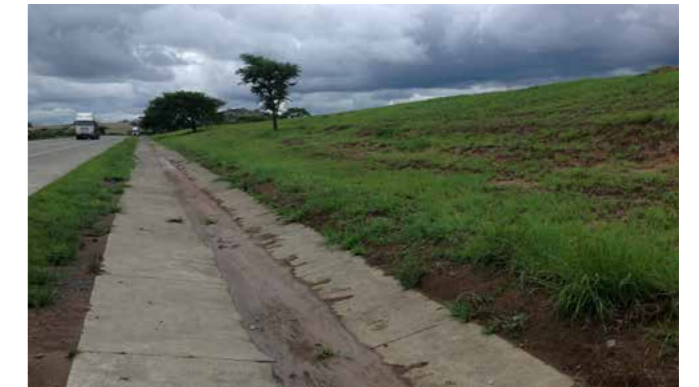
Photo 4: Steep cut embankments produce huge amounts of sediment – noticeable when the gradient in the gutter is low – which goes into the nearest watercourse.
