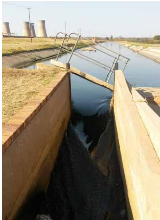
Partially treated sewage entering a small river from a hydraulically overloaded WWTW. (Image courtesy Anthony Turton)
