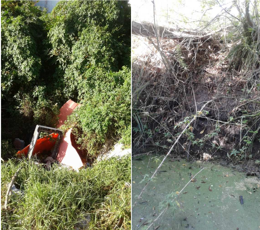
Picture 7: Open ditch, south end 3.5m deep and north end 1.5m deep
