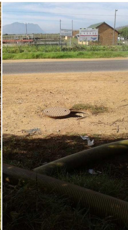
Sewer from Wetland side
